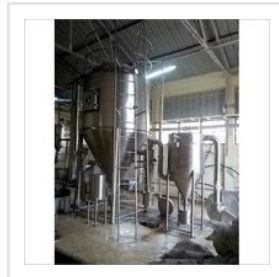
Pilot Spray Dryers
