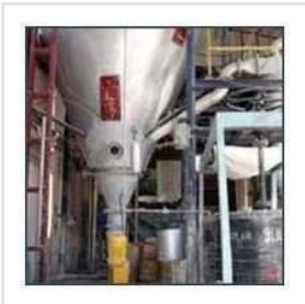
Spray Drying System
